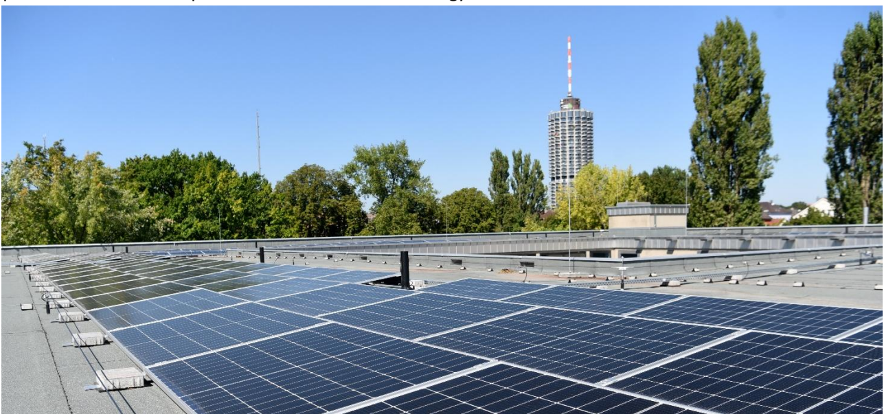
Photovoltaic system at the Gymnasium bei St. Anna grammar school (source: Ruth Plössel)
